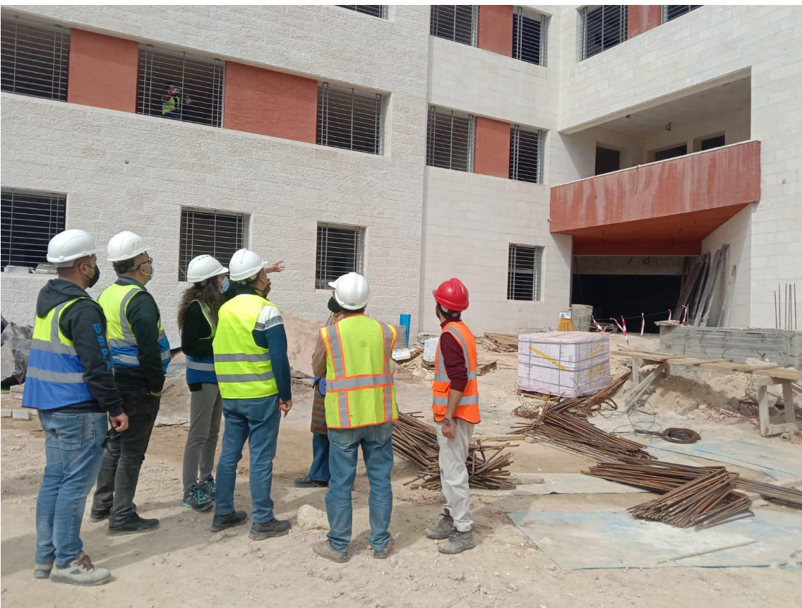
The team observed that there was a white color on the external top finish color resulted from other works and made a distortion to the original color. The team requested the Contractor to rectify as needed
