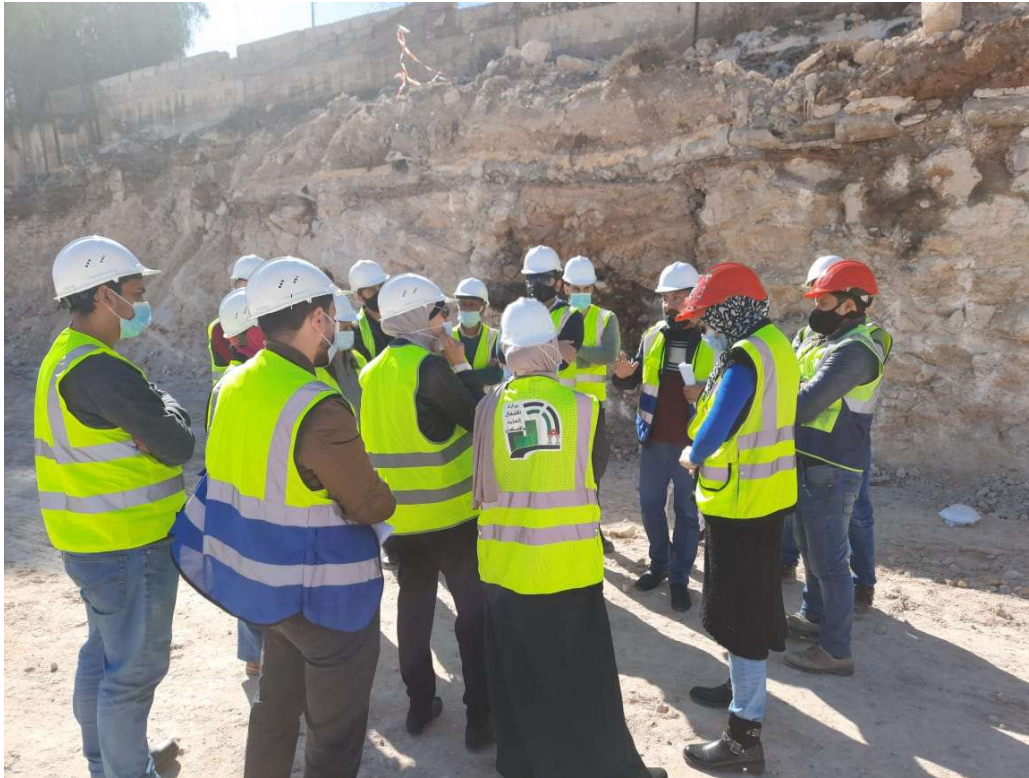
Eng. Basema from MPWH discussing the actual status of the North-East boundary wall with Medanat site staff
