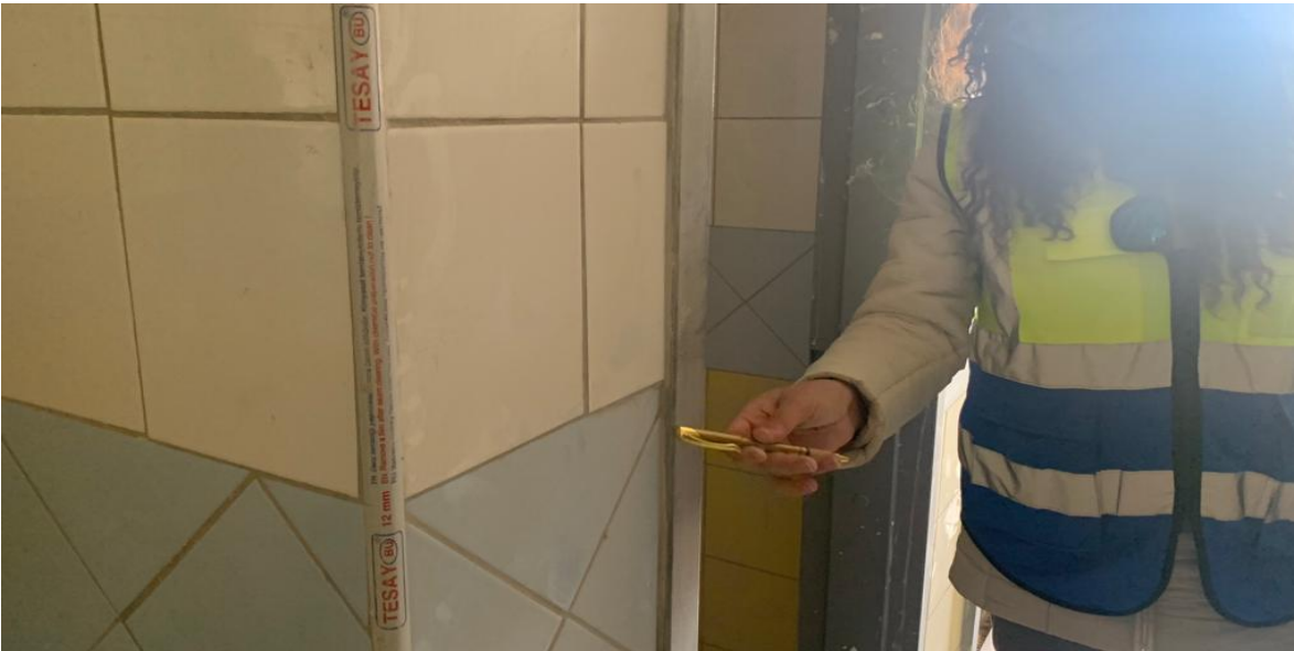
Defects in ceramic cutting adjoining the door frame
