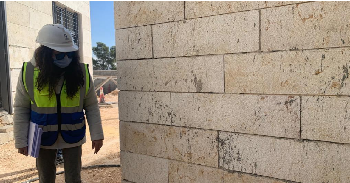
Defects in the built stones
