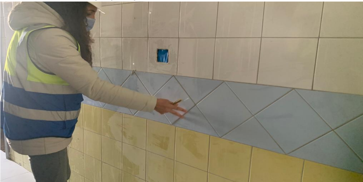
Teething and defects in grouting of the wall ceramic
