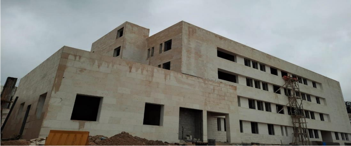
Defects in the built stones
