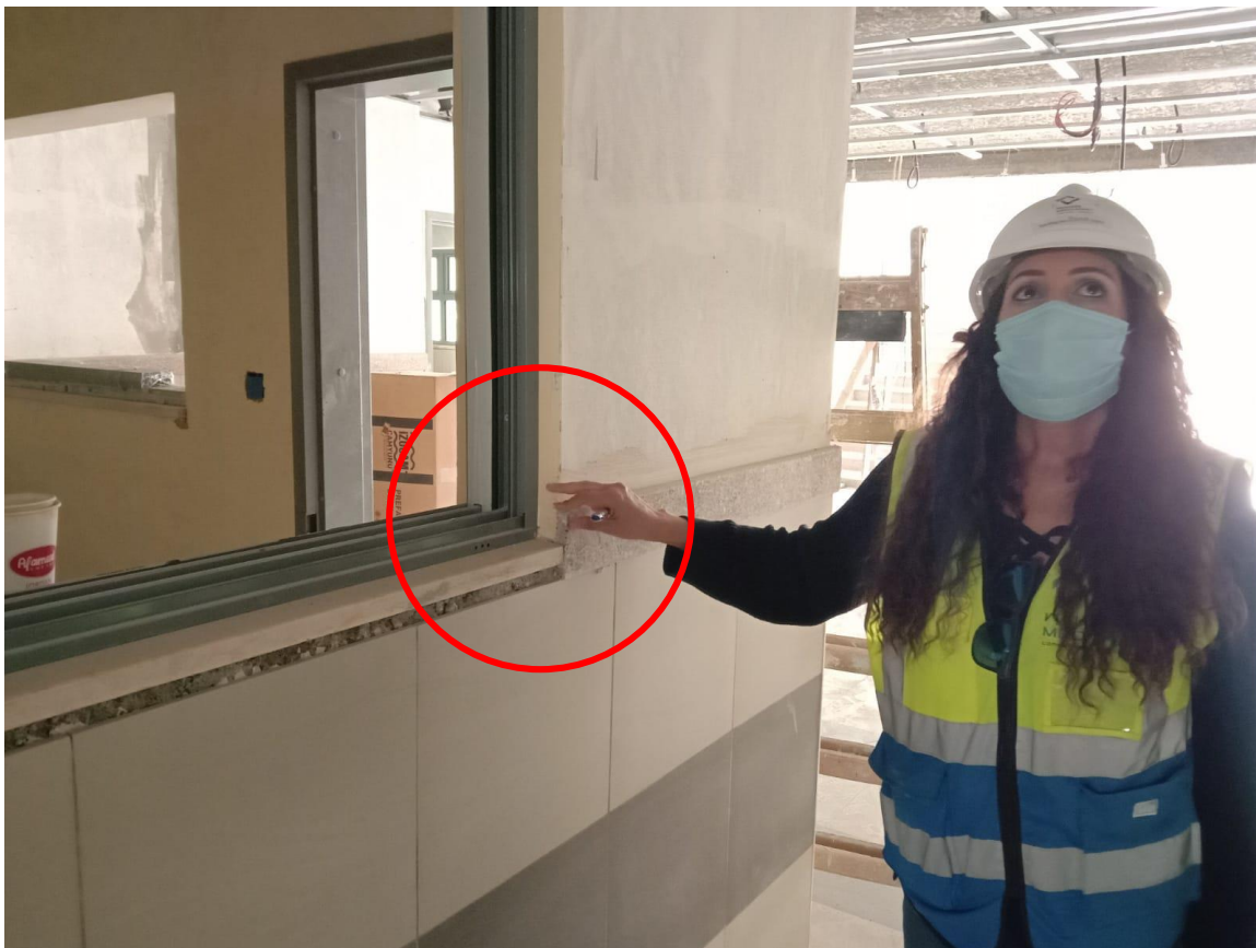
The team instructed the Contractor to extend the granite coping over the porcelain at corridors to be also at the window jambs using small pieces
