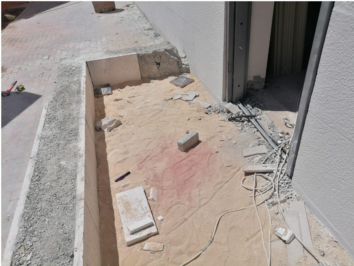
The team discussed with the Contractor the execution of ramp for the disabled at the multi-purpose hall emergency exit
