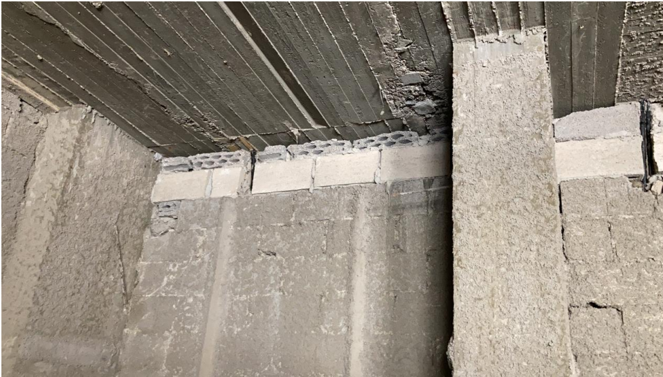
Blockwork: Top layers at same places are built incorrectly-need to be removed and re-built correctly and evenly
