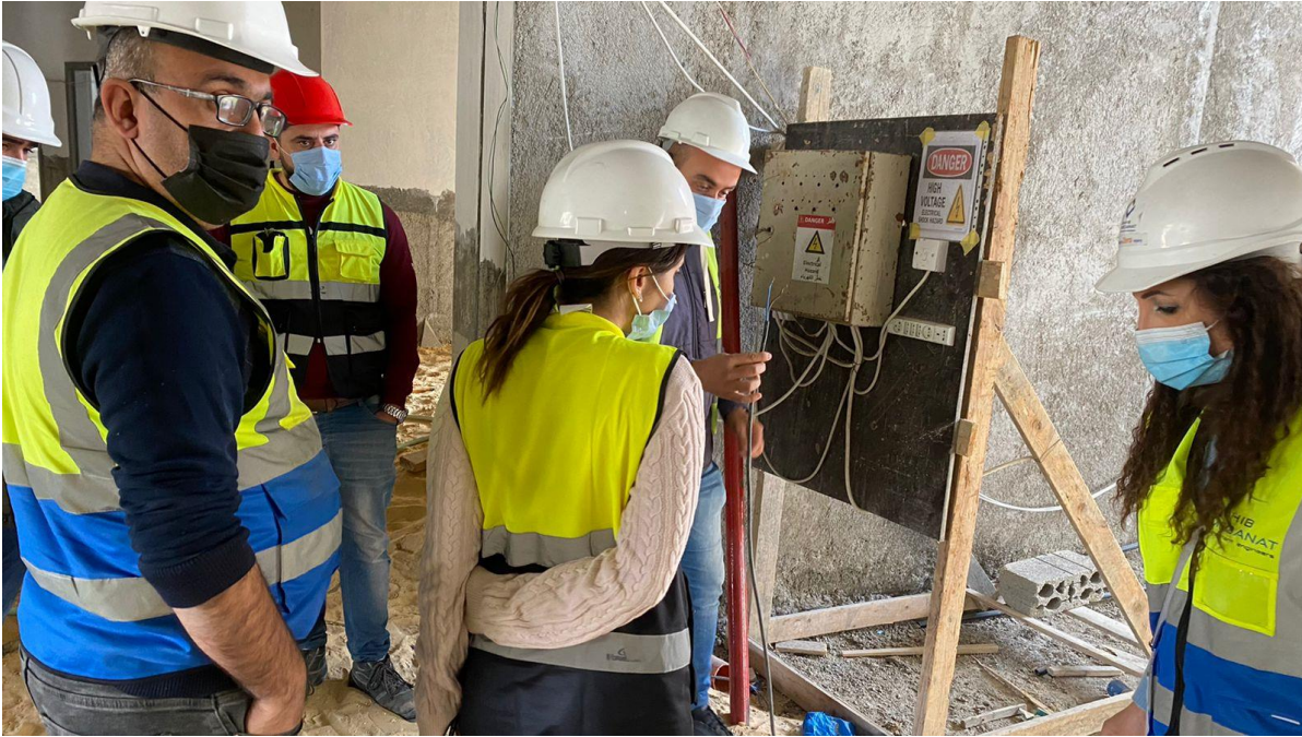
Eng. Natheer commented on the correct way of installing temporary electrical wiring inside the building
