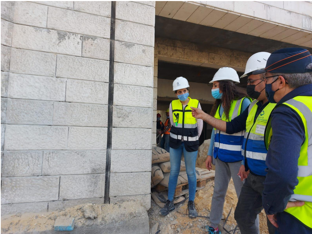
The Engineer presenting the Designer advice to keep the expansion joint as executed without fixing the aluminum cover. The details in the drawings should be taken into consideration
