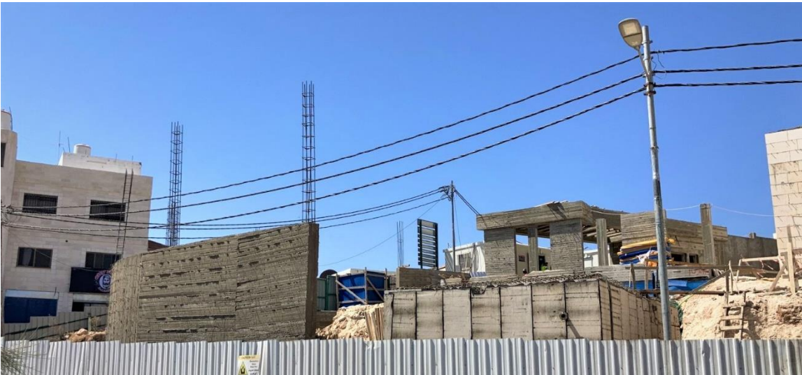
Executed part of the external works at the side of the street down which was delayed due to the encroachment inside the school plot
