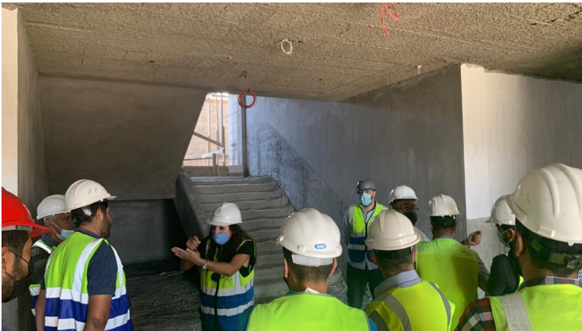
The Contractor was requested to submit shop drawings for the false ceiling at corridors to specify the details of the false ceiling end at the staircase areas
