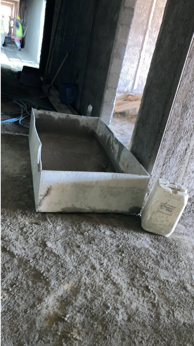
The Contractor is using a special container for mortar mixing used for plastering
