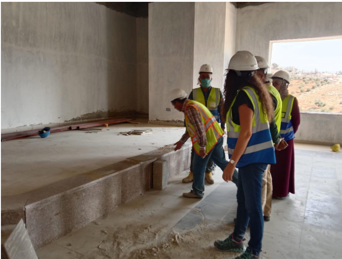
Granite cladding installation for the platform at the multi-purpose hall was inspected
