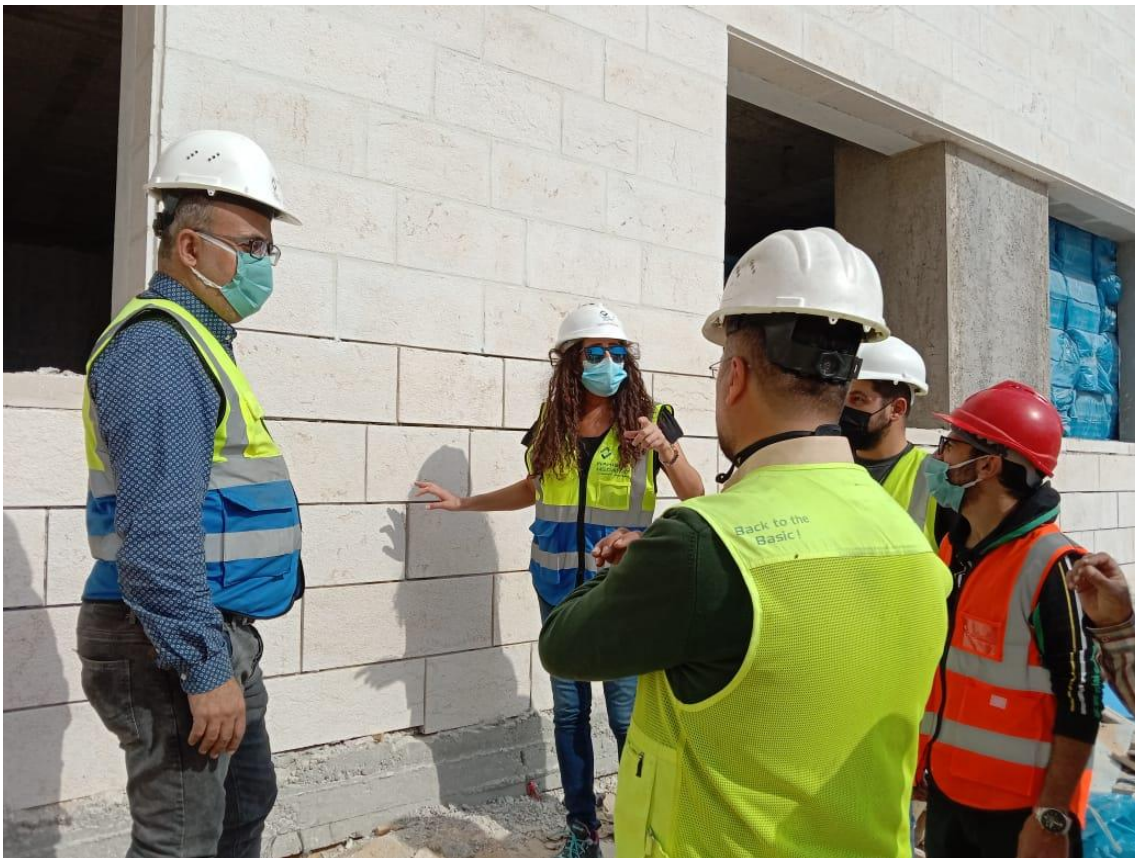
The stone work at the facades was inspected and the Contractor was requested to replace the defected and broken stones
