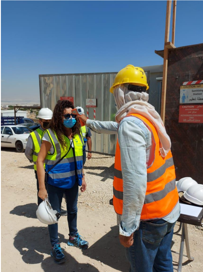
Temperature check, sterilization and signing visitors' attendance sheet at the entrance of the site, complying with Covid-19 Protocol
