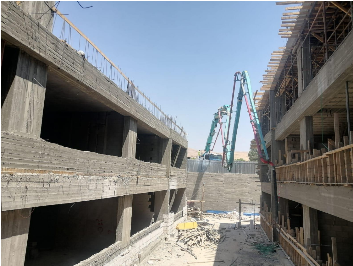
Backing concrete for stone façade has been witnessed at the ground floor between zone "A" and zone "B"
