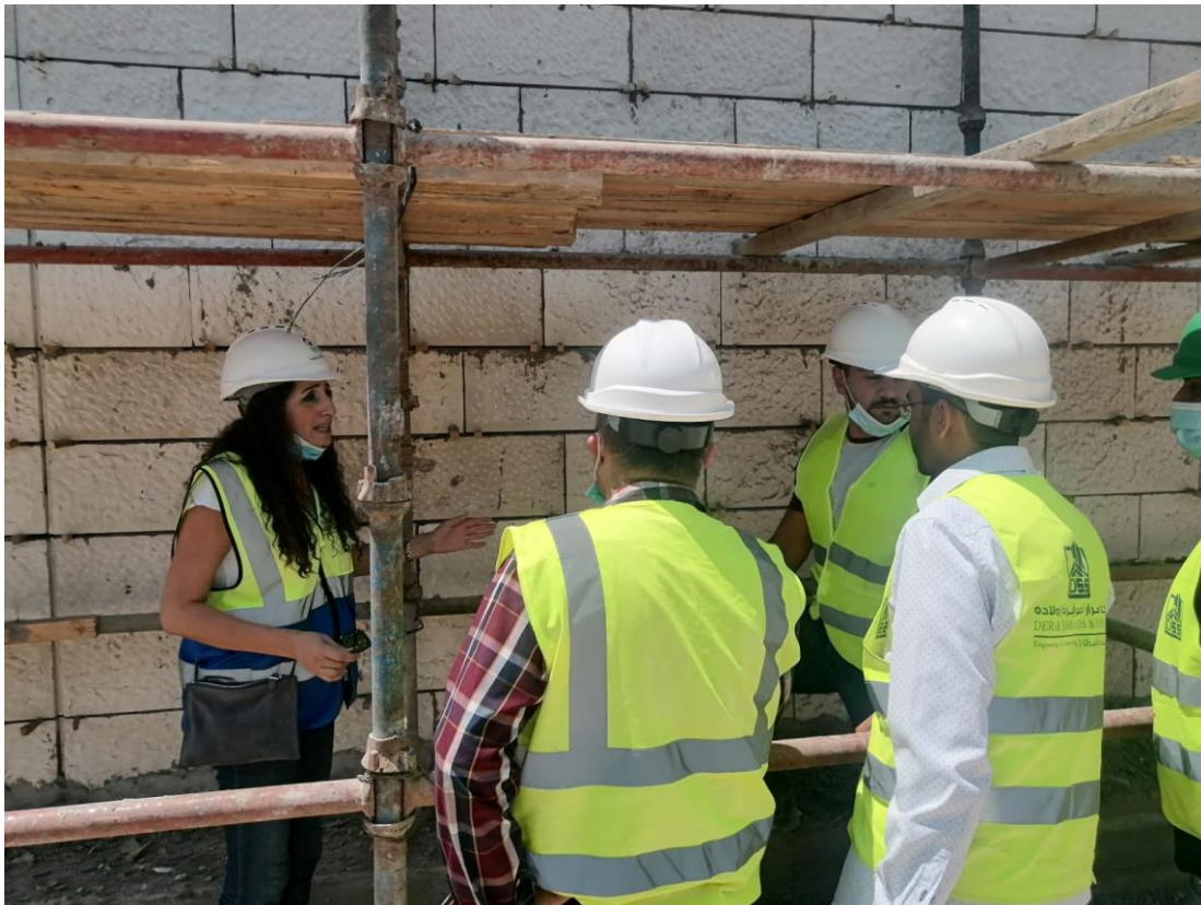
An inspection has been conducted on the built stones courses at the front and side elevations. Part of the built stones at the side elevations has been built without using the appropriate stiffeners for fixation
