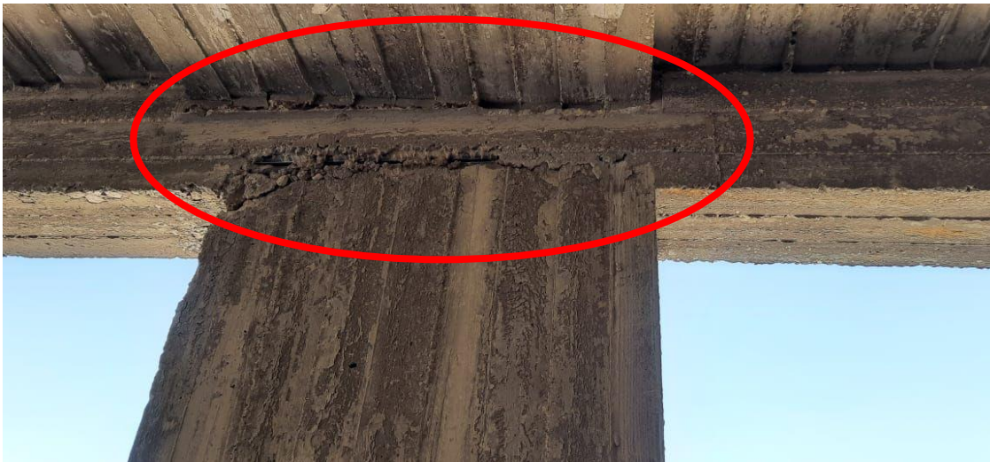
A roughness was observed at the soffit of the lately casted third floor slab. The Contractor was instructed to remedy the observed parts and any similar parts
