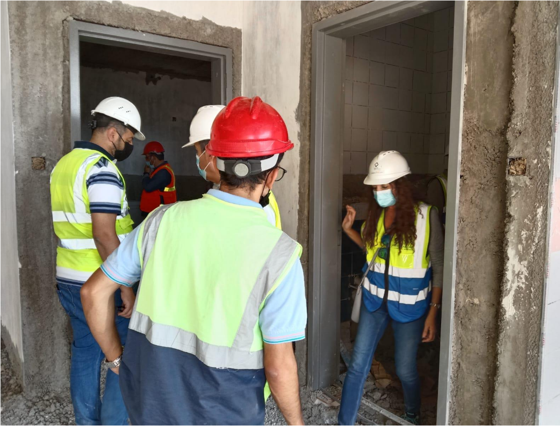
The installed steel door frames were checked and the Contractor was requested to protect those frames from any defects during the construction work
