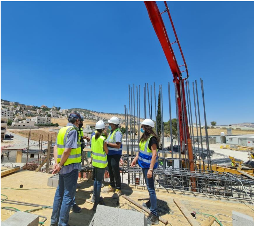
Discussing the distribution of bottom steel bars for ground floor drop beams/ground floor slab at zone A
