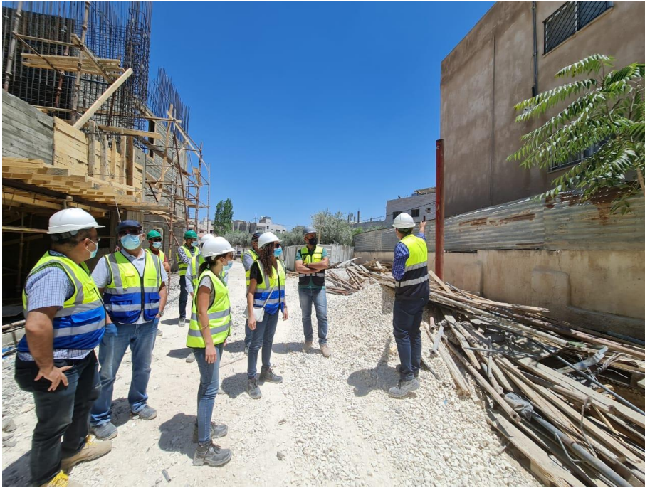
Checking the encroaching neighbor's building on the south-west side of school plot limits
