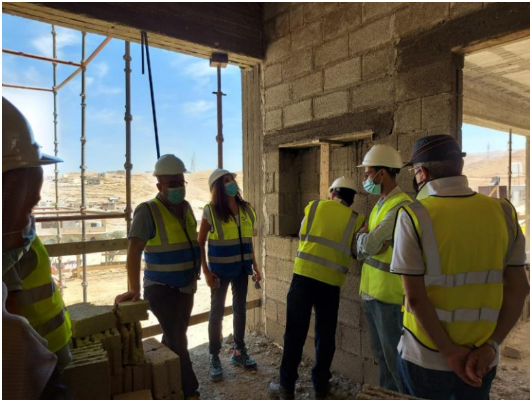
One location of "Fire Hose Rail Cabinet" was checked and remarks were given to Contractor regarding the finishing of the double wall
