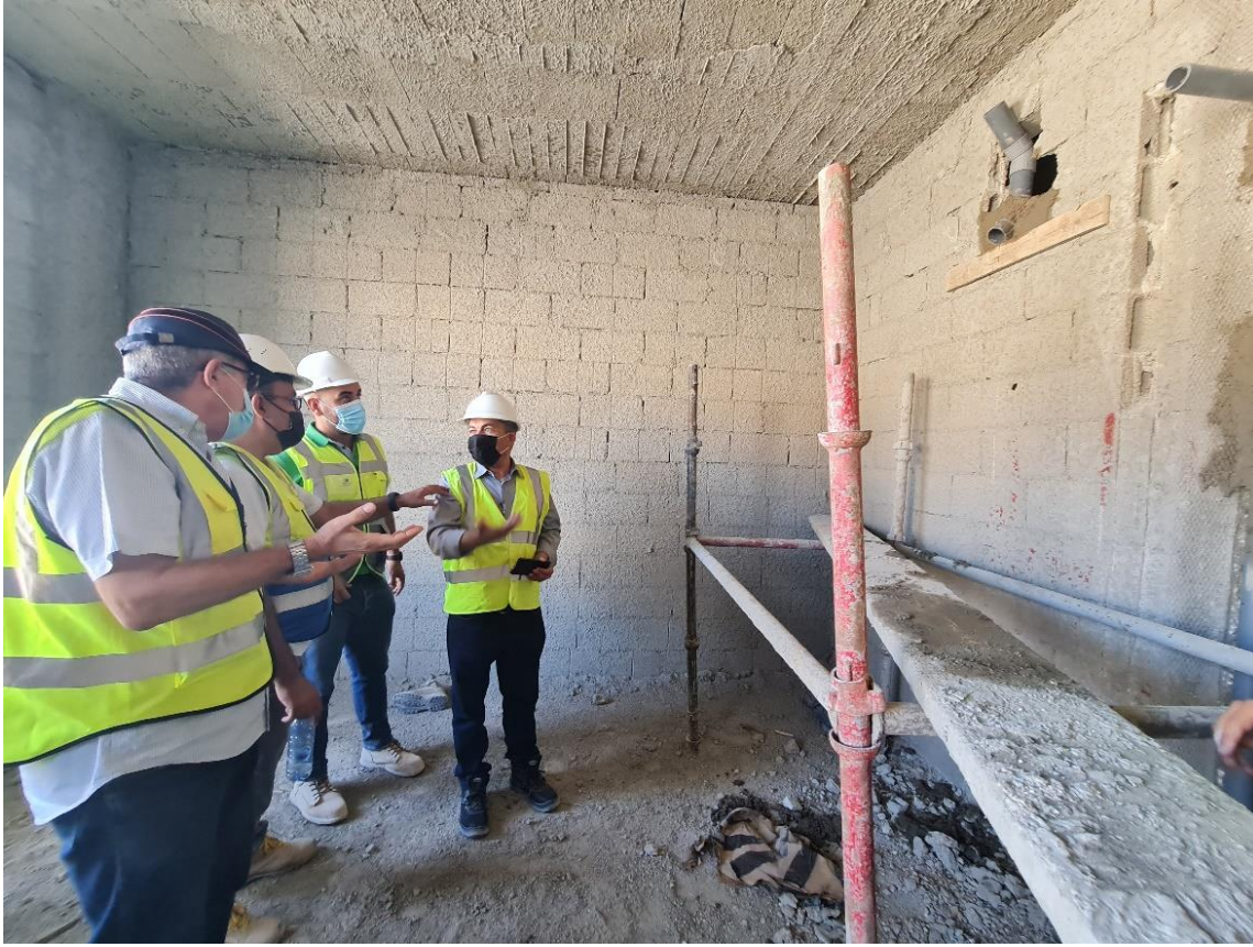
The level of sleeves for A/C and the relation with the false ceiling level were discussed
