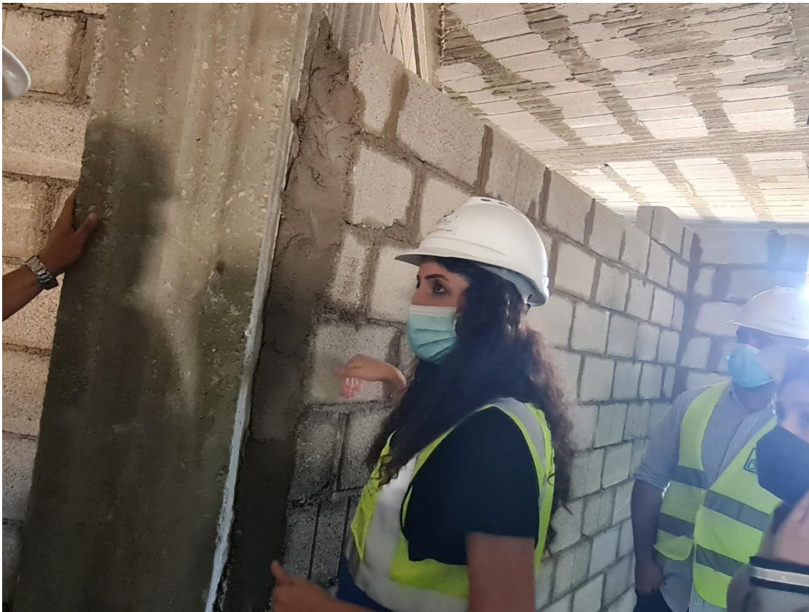
Engineer representatives requested that the inclined block wall at the corridor in the basement floor should be flushed with the column to avoid double angles
