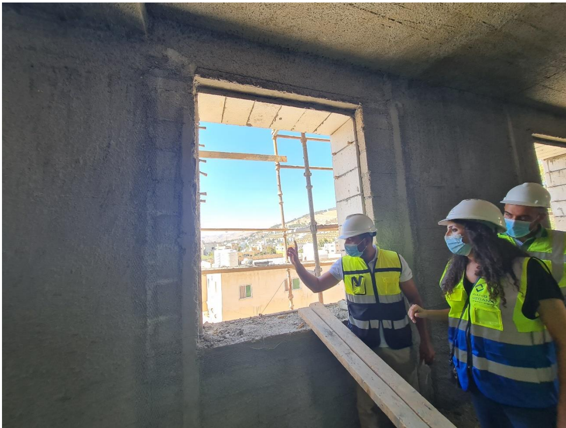
The erection of stone for the window frame at the top and for the two sides were discussed
