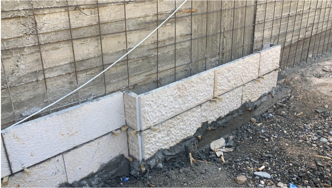
An example of stone work complying with the approved sample and specifications
