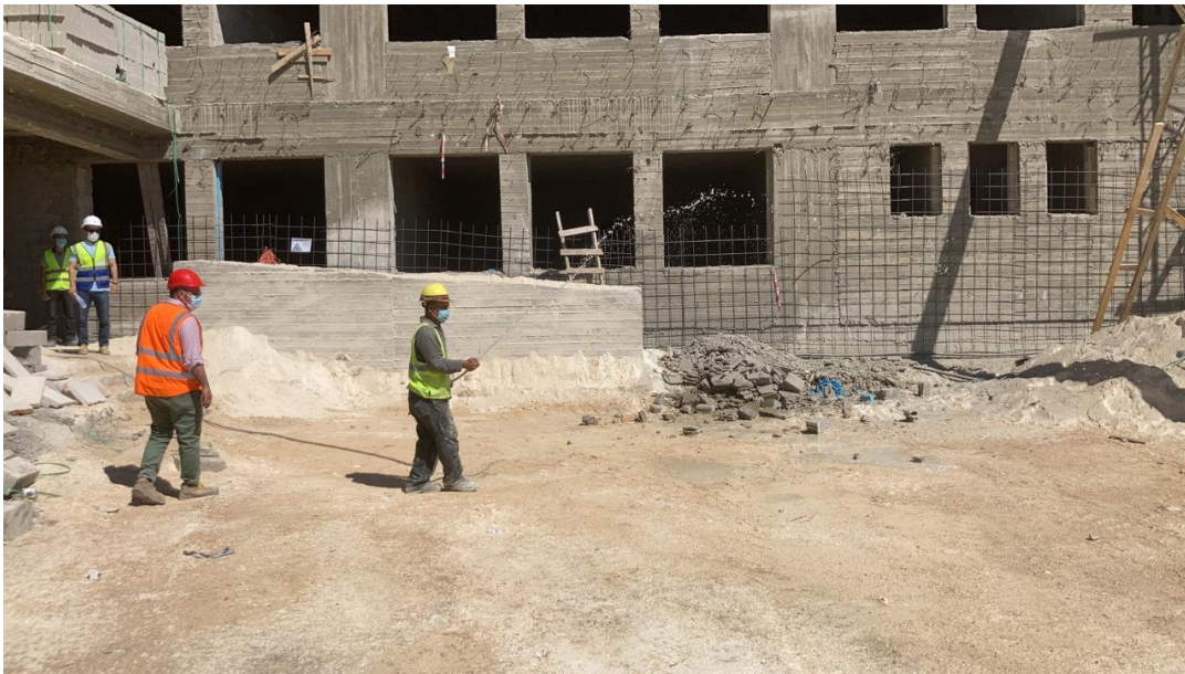
Spraying water at the sand areas in the site for the purpose of dust control
